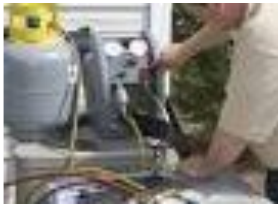
HVAC Service Technicians Training for Veterans
